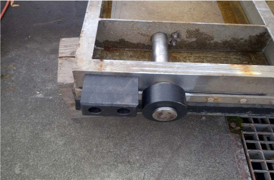
New entrance weir E2 plastic wheel and added rub block to assure alignment.
